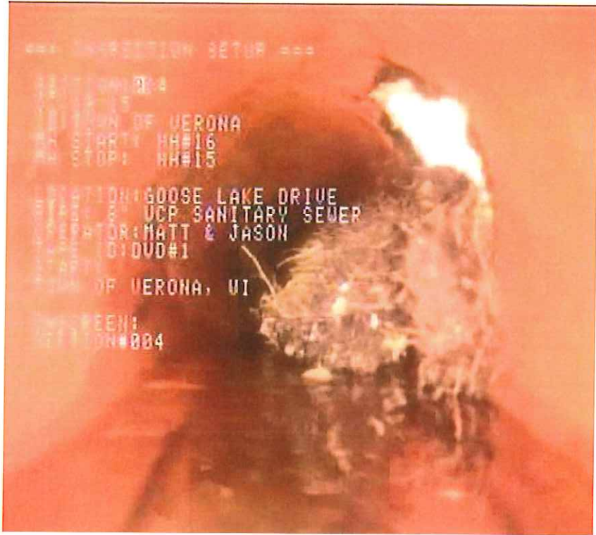
Roots in pipe 11 feet downstream from MH 16. Situated at existing tap
